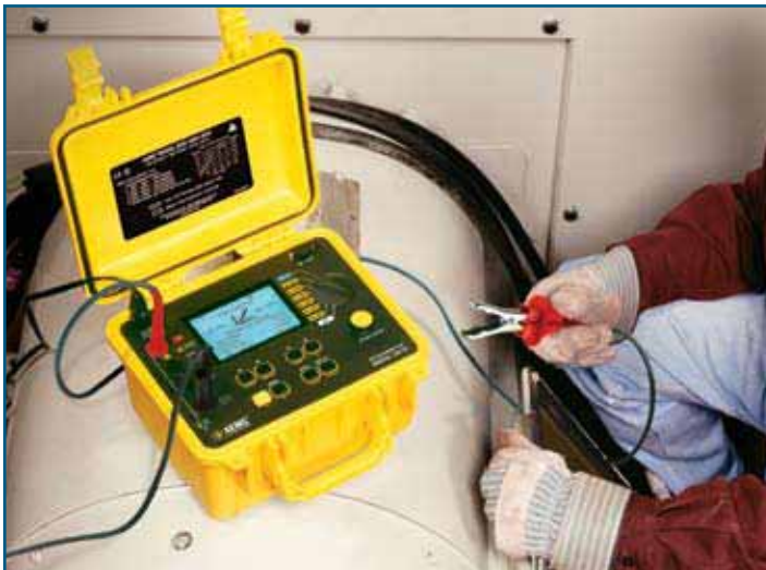
Model 5070 performing insulation test on a generator.
