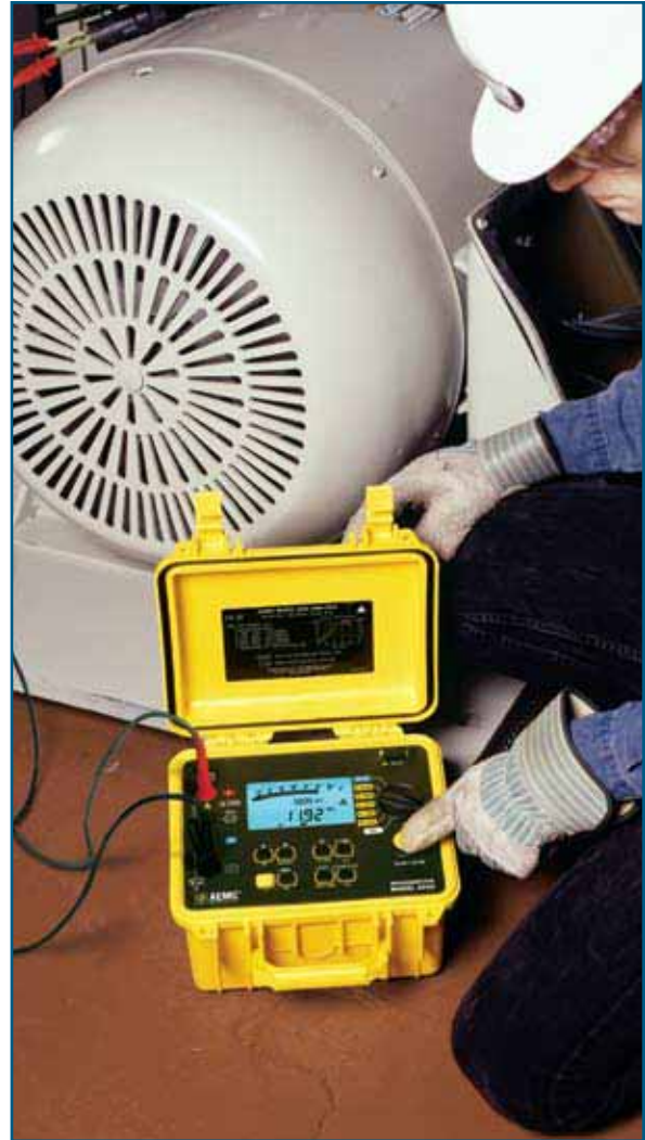
Model 5060 checking insulation resistance on feed cables to a three-phase motor.
